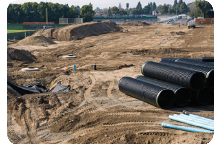
Industrial Technology/Athletic Fields: $24.7 million; 35,000 sq. ft.; expected completion is spring 2014. Includes new athletics facilities: baseball field opens Jan. 26, 2013; football/track and soccer fields open summer 2013.
