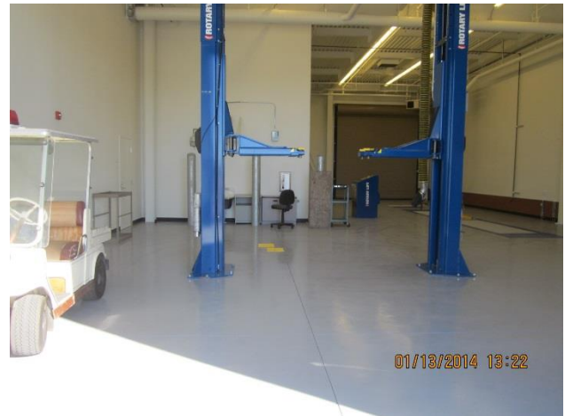
Vehicle Lift at Bldg. 2
