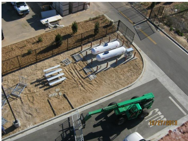
Fire Tower – Propane Tanks
