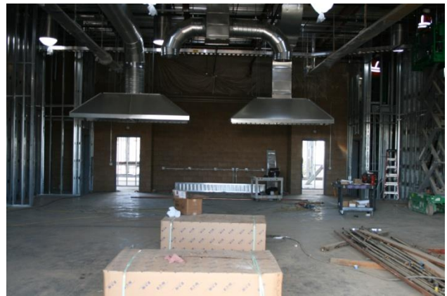
Mechanical Hoods at Building 0-200 Welding Lab 2
