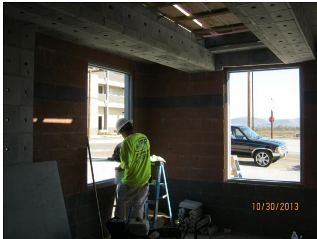
Class A Burn Bldg. High Temp Lining
