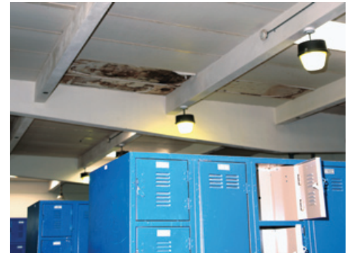
Building N, locker room ceiling
